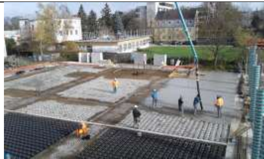
The Slim-Line void formers on the ground floor slab of the project “Zielstattstraße 27” being concreted.
